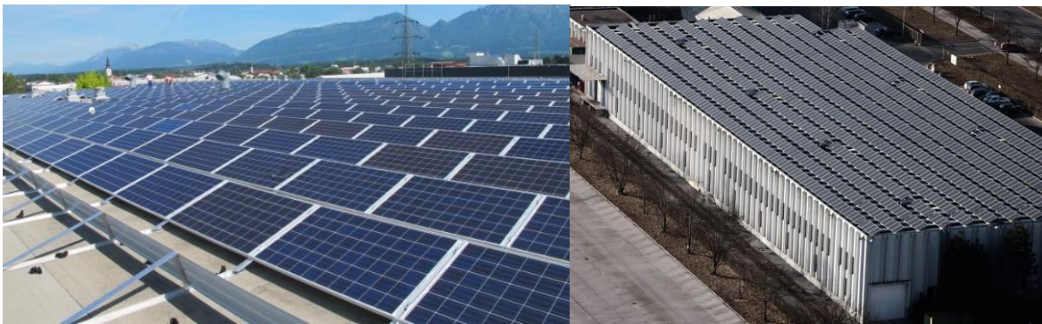
Figure 15: Solar power plant on the roof of the Merkur's warehouse in Naklo (left) (Merkur-nepremičnine, n.d.) and solar power plant on the roof of BTC (right) (Ba. P., 2011).
